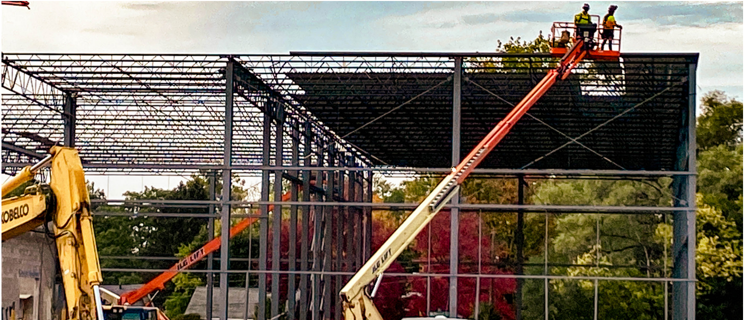
Work continues on Cultivate Culinary's Cold Storage Facility. Cultivate was the recipient of a $250,000 Special Project Challenge Grant this spring.
